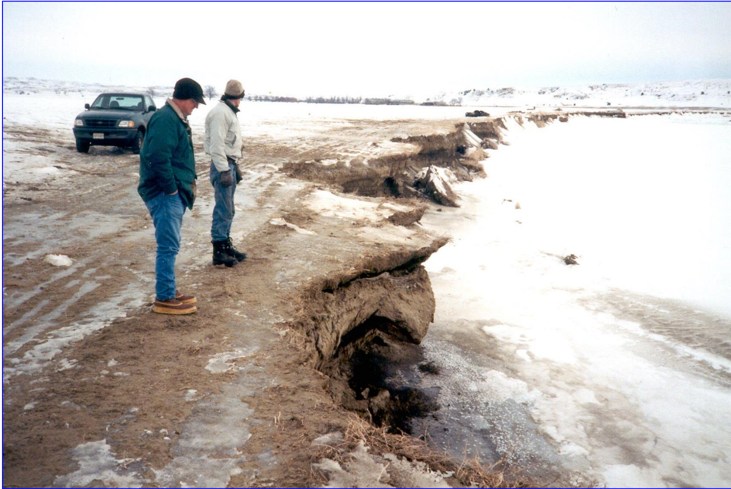
Perplexed ranchers viewing wintertime, bank erosion along Missouri River, Eastern Montana (a reach d/s of Ft Peck Hydro Dam)
